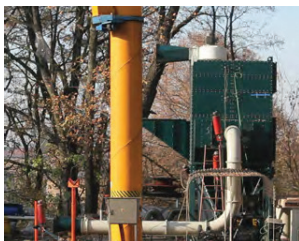
At the start up of a staged explosion, explosive dust is injected into the dust collector to create a flammable cloud.
