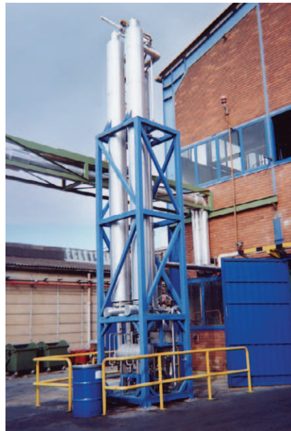
Cryogenic Condensation Unit – Installation 1
