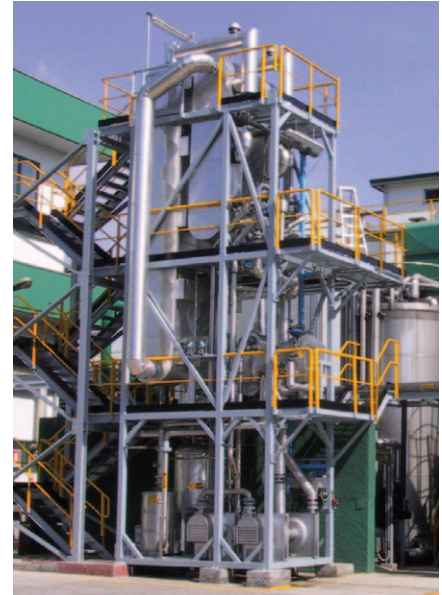
Cryogenic Condensation Unit – Installation 2
